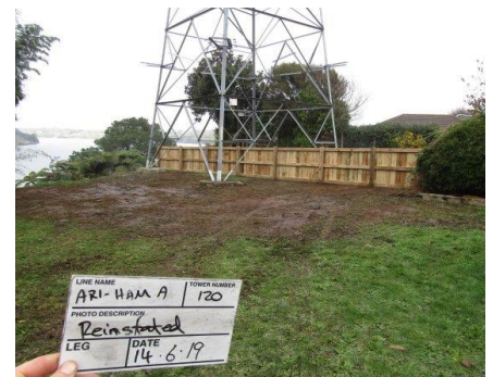
Tower (after) with foundations completed and wooden fence replacement, prior to grass regrowth.
