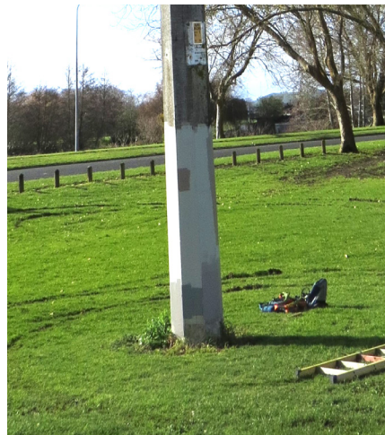
Pole (before) in a park reserve.
